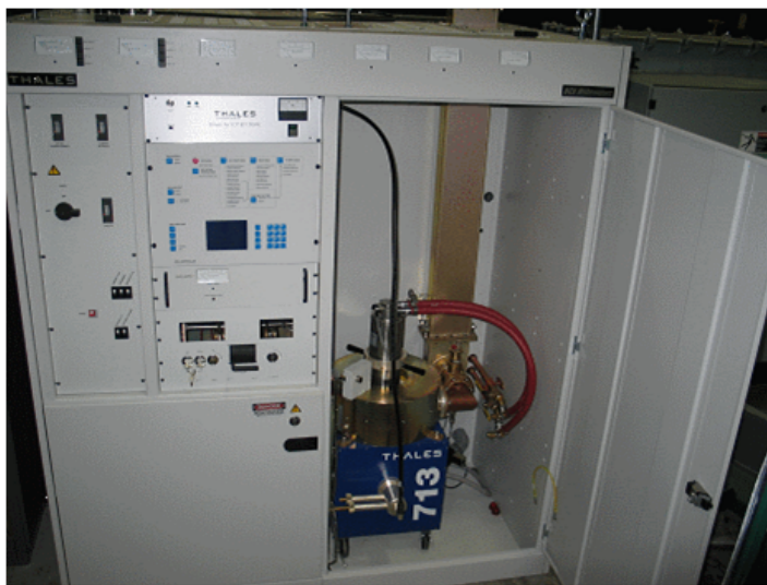
Figure 4.5.3: IOT inside the transmitter.
