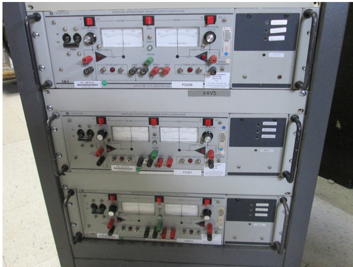
Figure 3.4.1: The front panels of the Kepeco Supplies.
