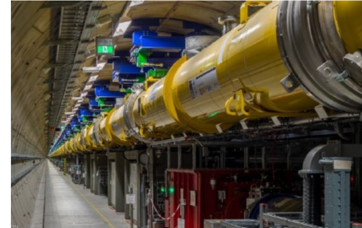
Installed cryomodules in the European XFEL
